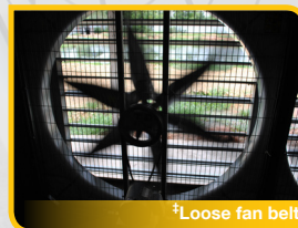
‡ Loose fan belt
